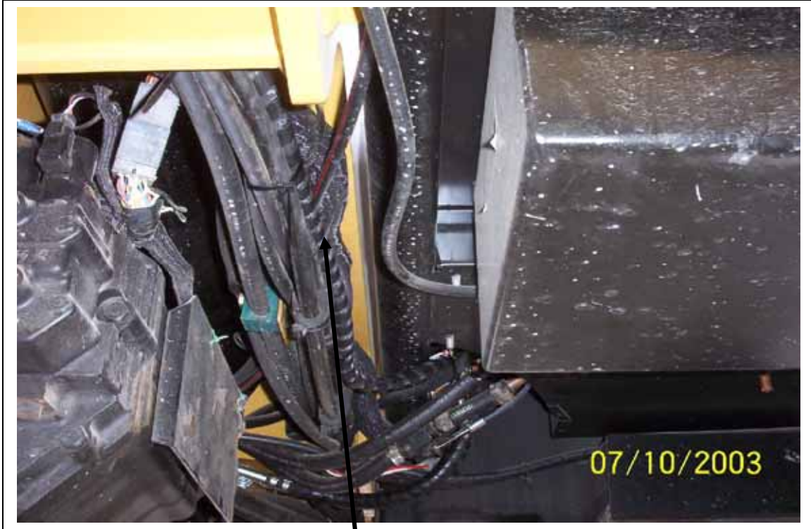
5/16" hose running between the drier and the expansion valve.
