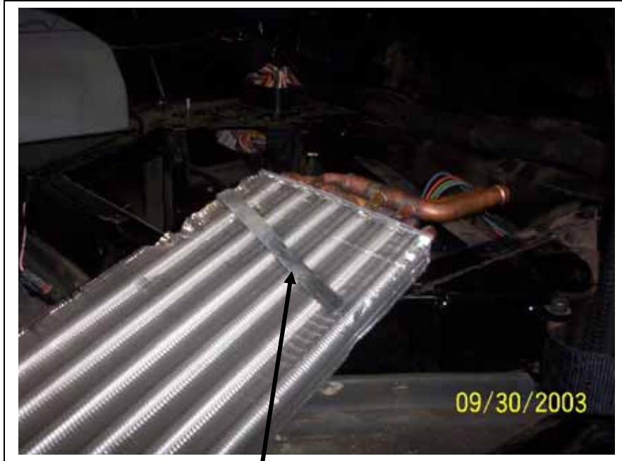
Flange removed from the coil.
